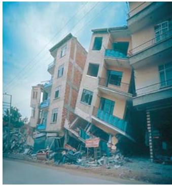
Fig. 4 Sway mechanisms with soft storey ground floors (Izmit, Turkey 1999)
