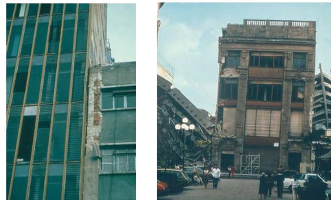
Fig.16:- Pounding damage of adjacent buildings
