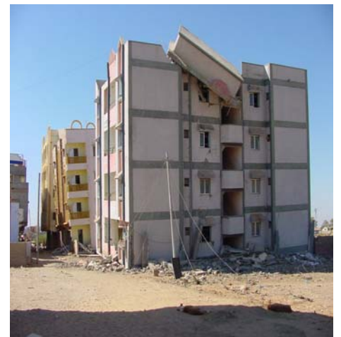
Fig.10 5 storey R.C., collapse of open plinth, water tank at top dislocated (Bhuj)
