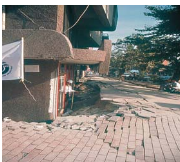
Fig. 1 The Building Sank evenly about 1 m due to soil liquefaction. The displaced soil caused a bulge in the road.
